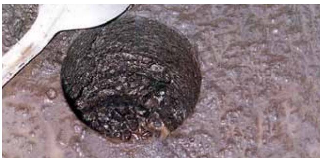
Figure 10: Photo showing the loss of bond between aggregate and binder leading to the commencement of asphalt stripping within this core hole
